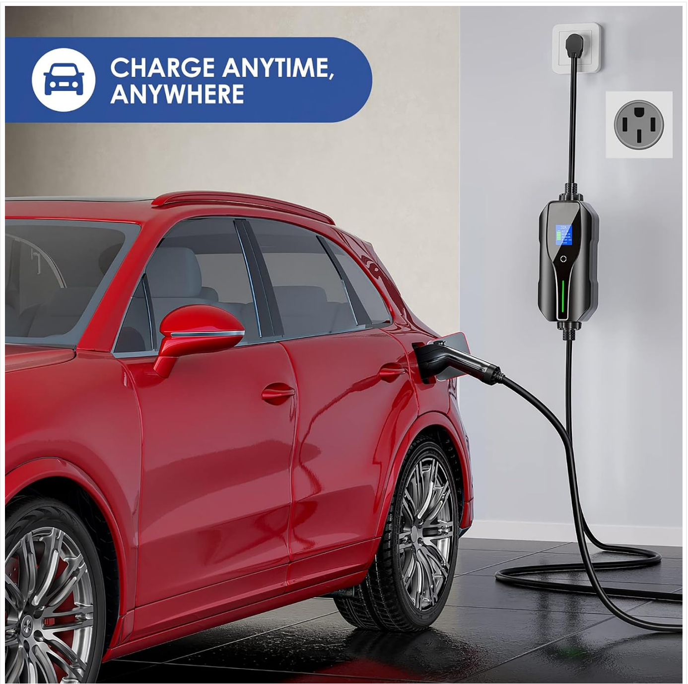
Figure 4.2: Example of the EV charger installed on a wall for convenient home charging.
