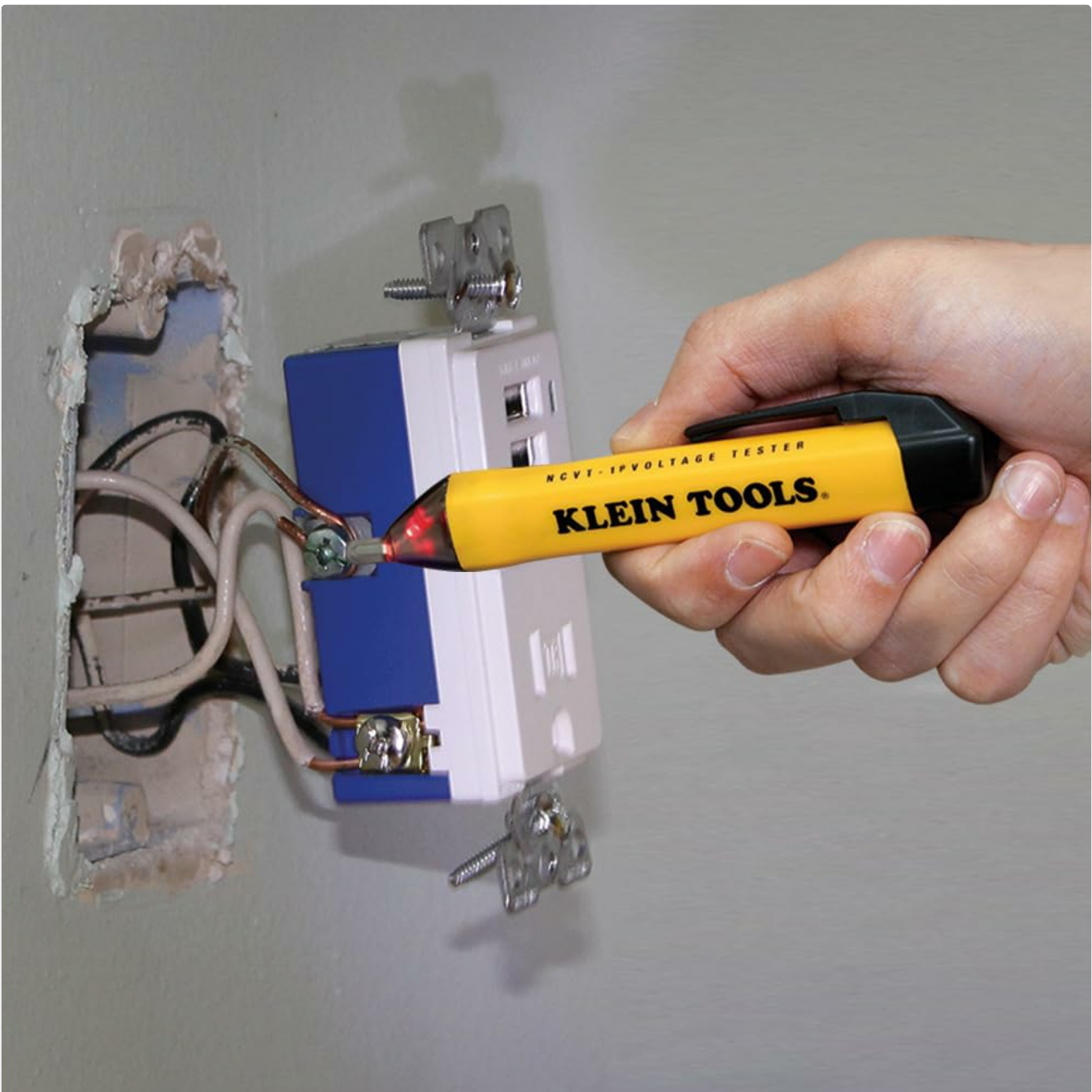
Figure 6: NCVT1P in use, detecting voltage at an outlet.
