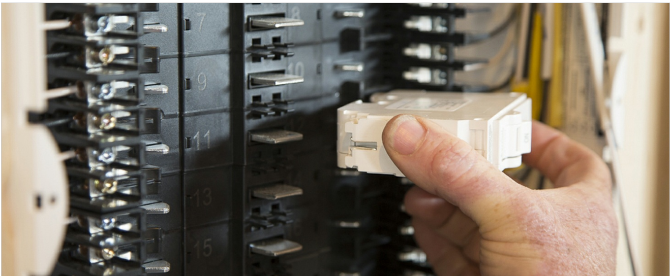
Figure 4.2: An example of a Leviton Load Center with neatly organized wiring, utilizing the integrated cable tie notches.
