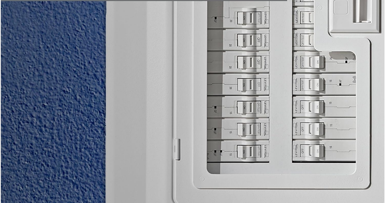
Figure 5.1: Close-up view of circuit breakers within the load center, visible through an observation window in the cover.
