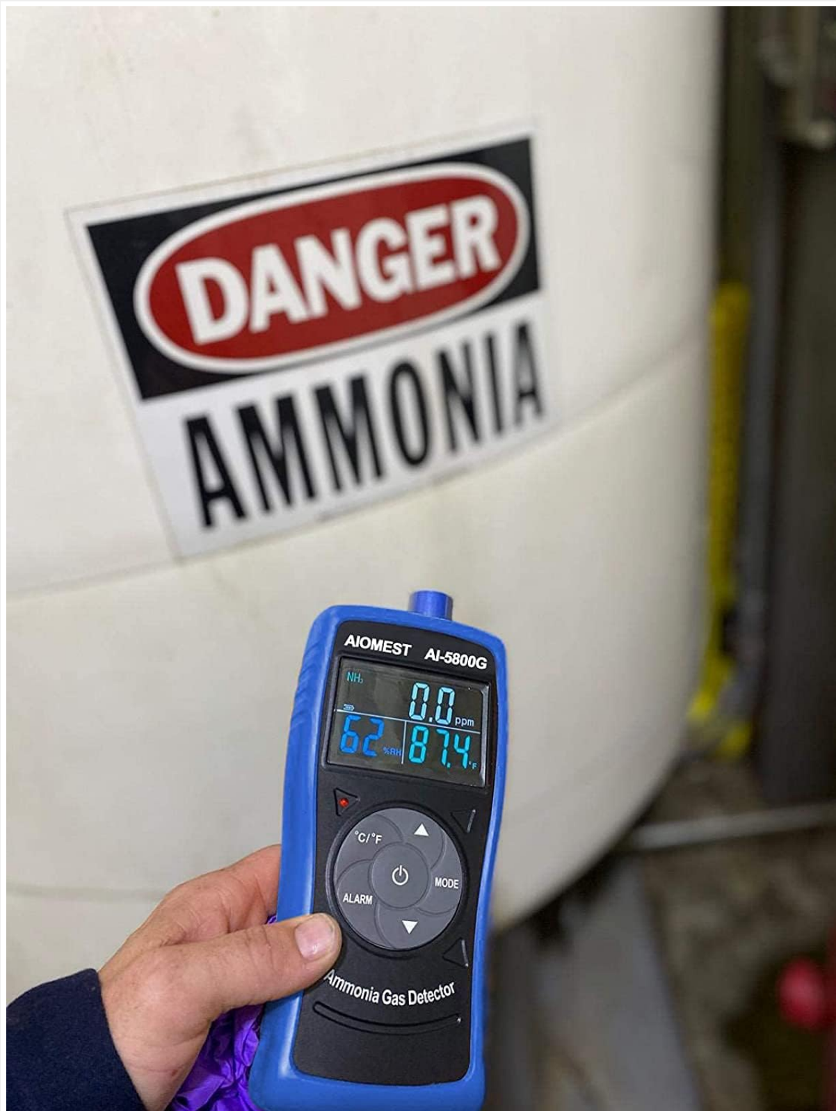
Figure 8.1: The detector being used in an environment with a "DANGER AMMONIA" warning, emphasizing its role in safety.
