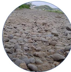
Uneven & Irregular Road
