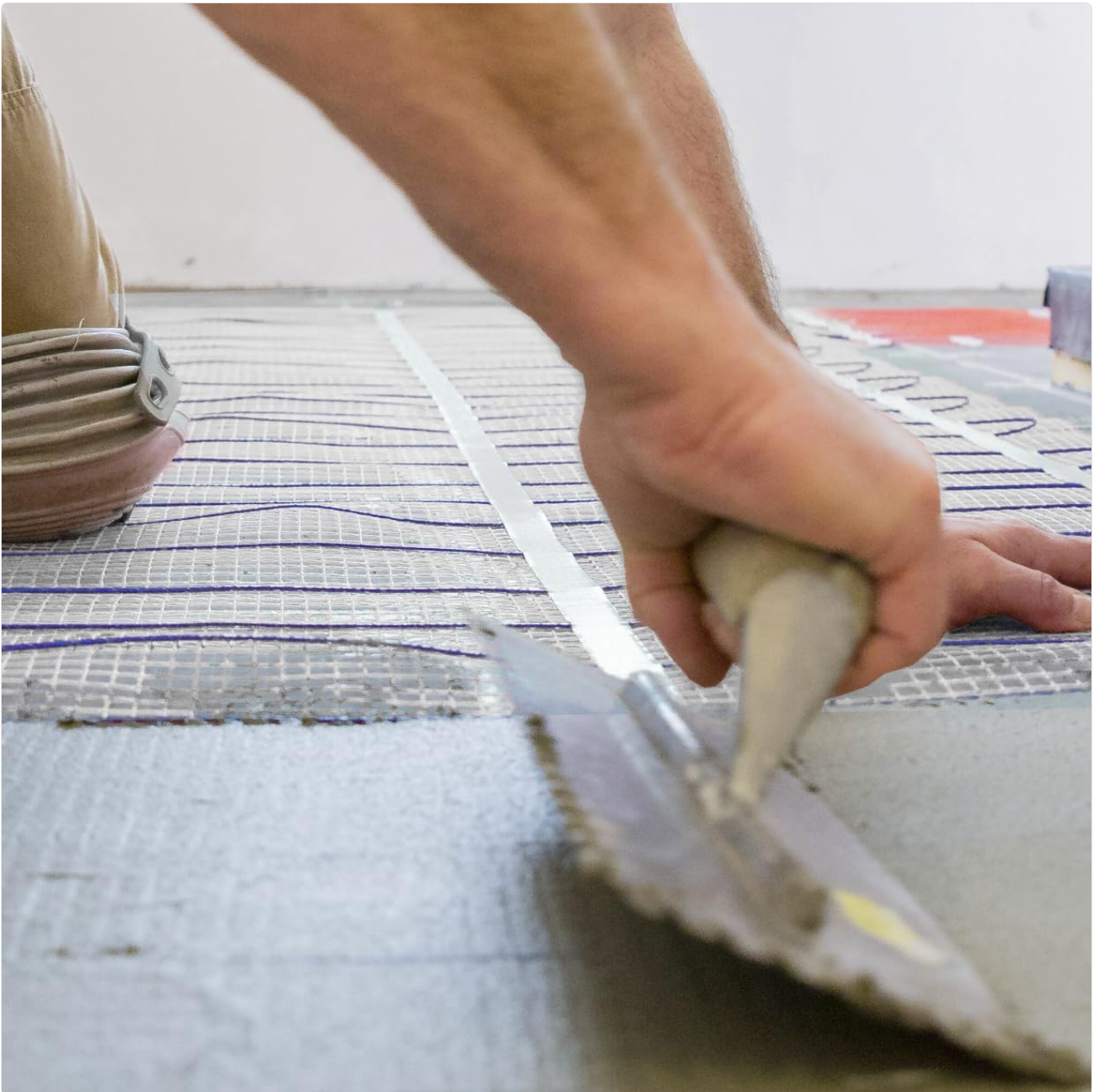
Image: A worker applying tile adhesive over the installed Rointe Milos heating mat, ensuring full coverage of the heating elements.
