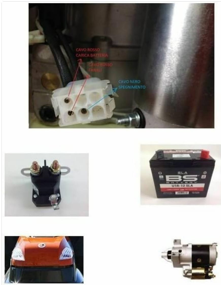
Figure 3.3: Electrical connector showing wire assignments: Red wire for battery charging, Red wire for lights, and Black wire for engine shutdown.
