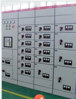
✓ High and low power distribution cabinet
