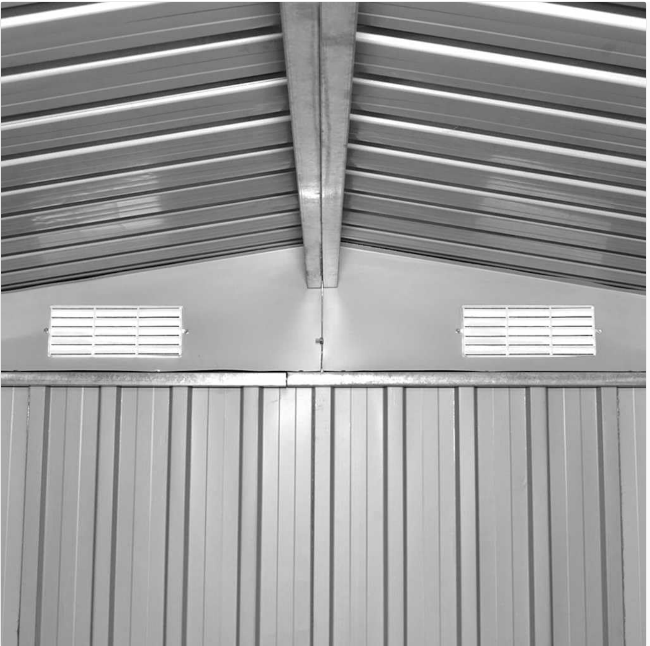
Figure 6: Interior view showing the roof structure and one of the ventilation openings.
