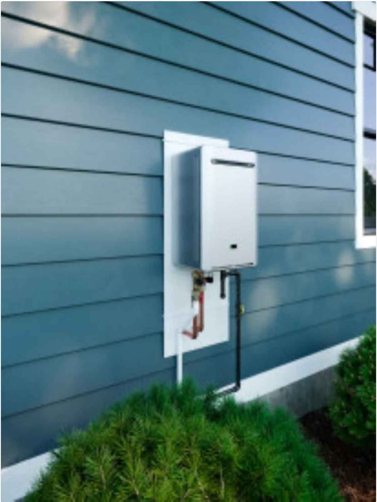
Figure 3: Example of an outdoor installation.
