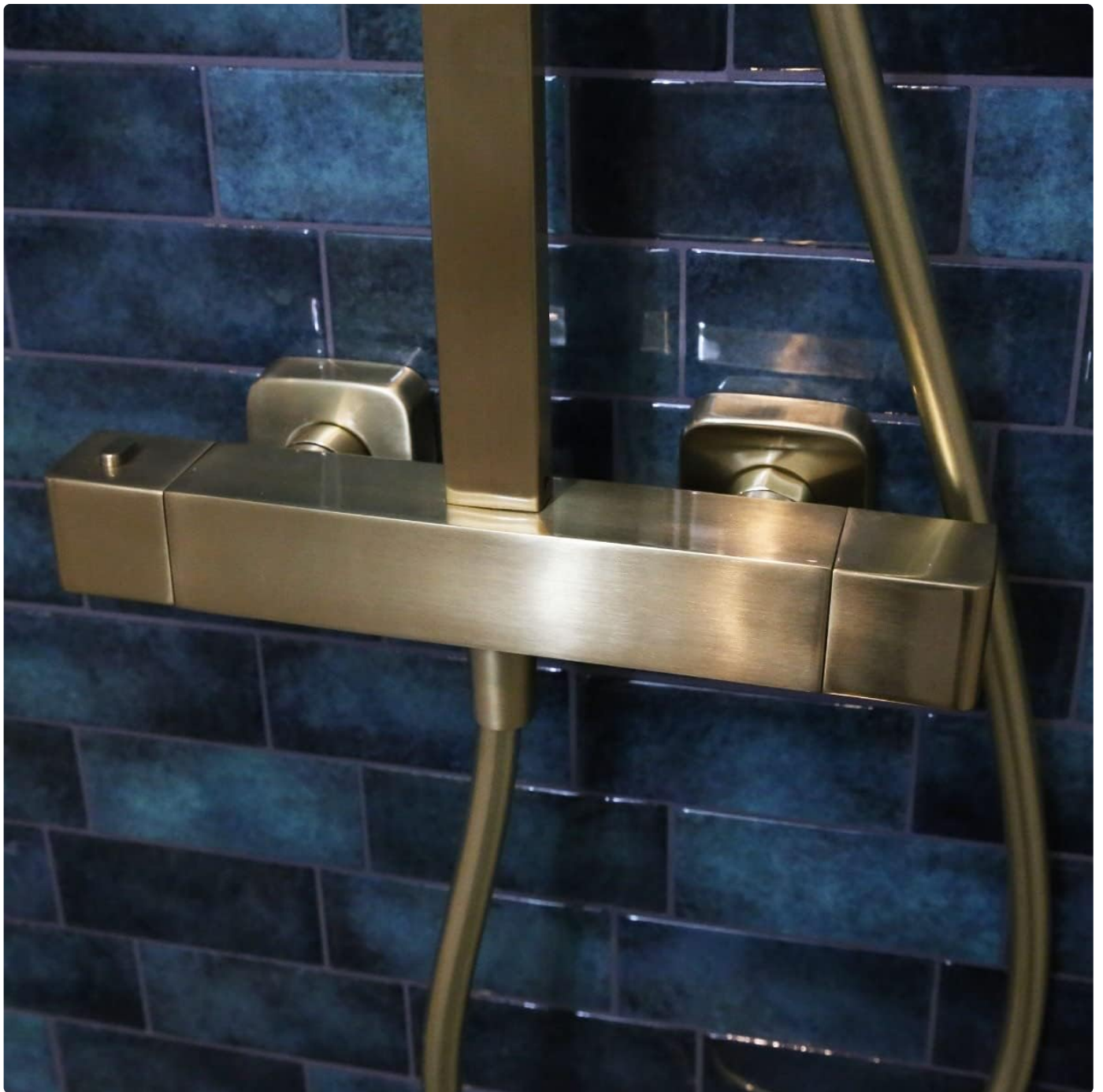
Image 6.2: The main thermostatic mixer unit, showing the two control handles for temperature and water flow/outlet selection.
