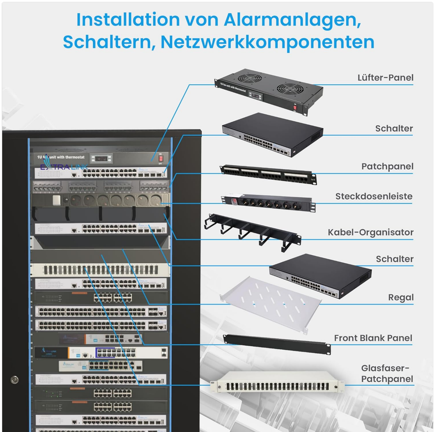
Figure 4: Example installation of various network and server components within a rack.
