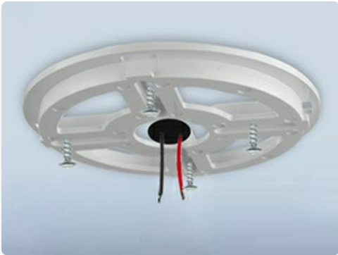
Image: Mounting bracket with wires exposed.
