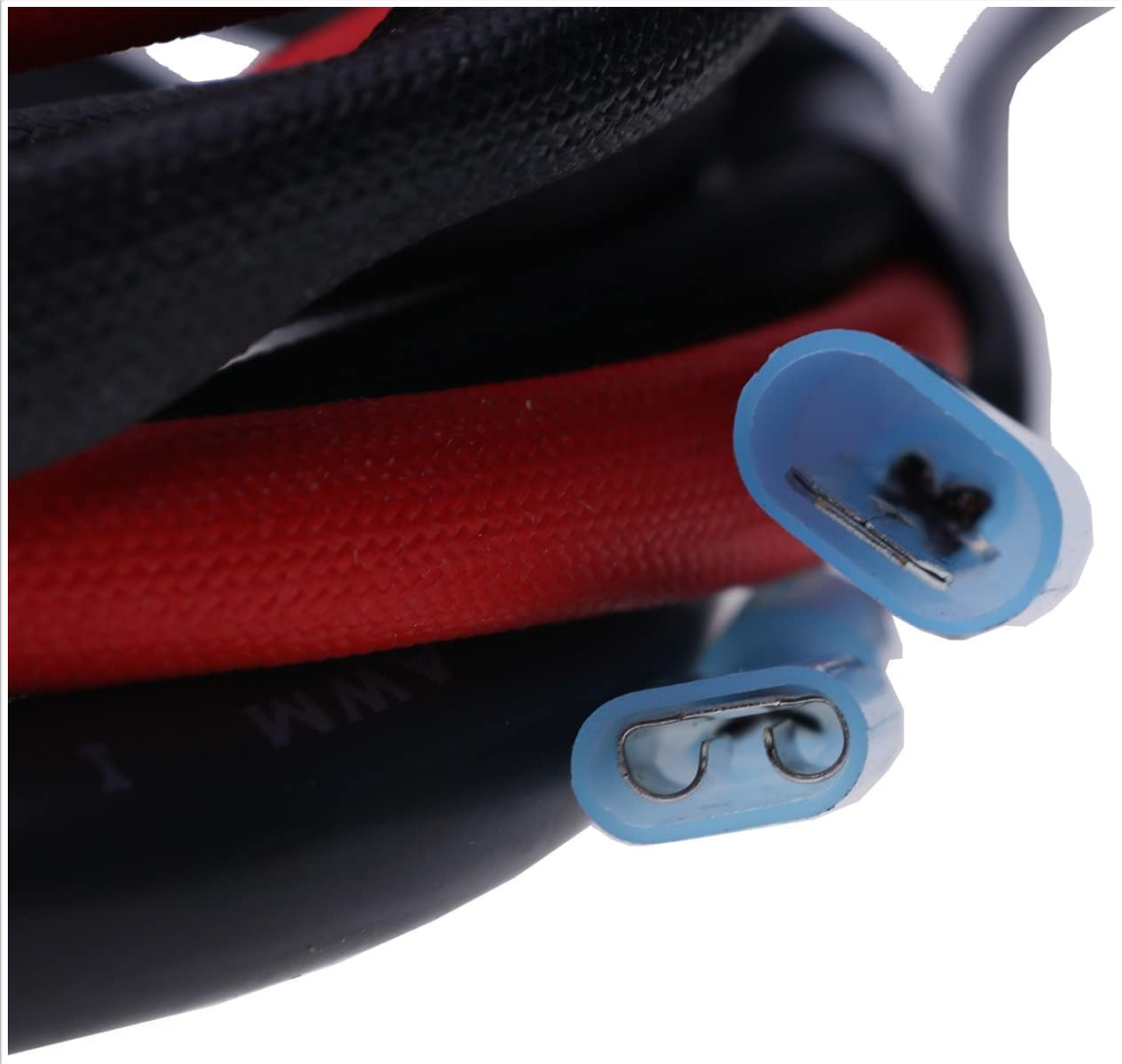
Image 3: Close-up view of the blue spade connectors on the interlock cables, which are used for integration with the lift's control system.
