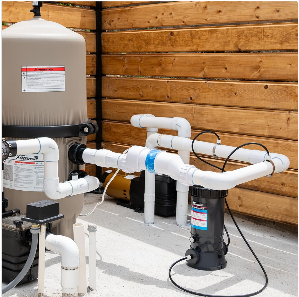
Image: An overview of a complete pool filtration system, including the pump, filter, and the XtremepowerUS salt chlorinator integrated into the plumbing lines.
