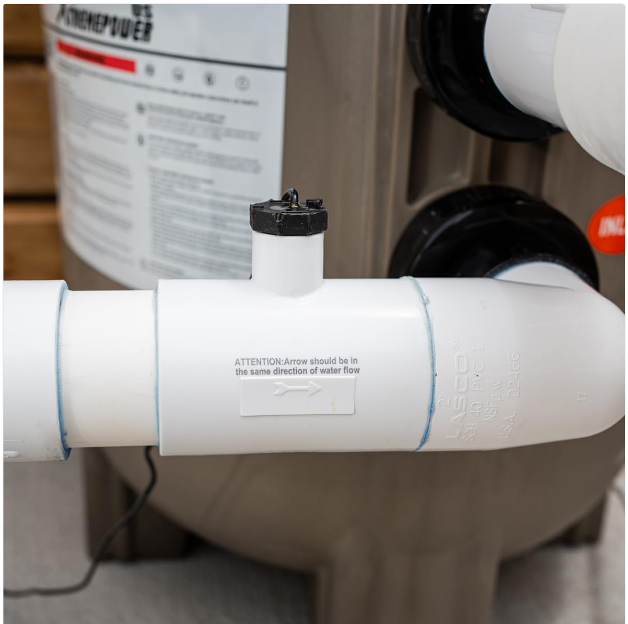
Image: A white PVC pipe section with a black flow switch installed, clearly showing an "ATTENTION: Arrow should be in the same direction of water flow" label.
