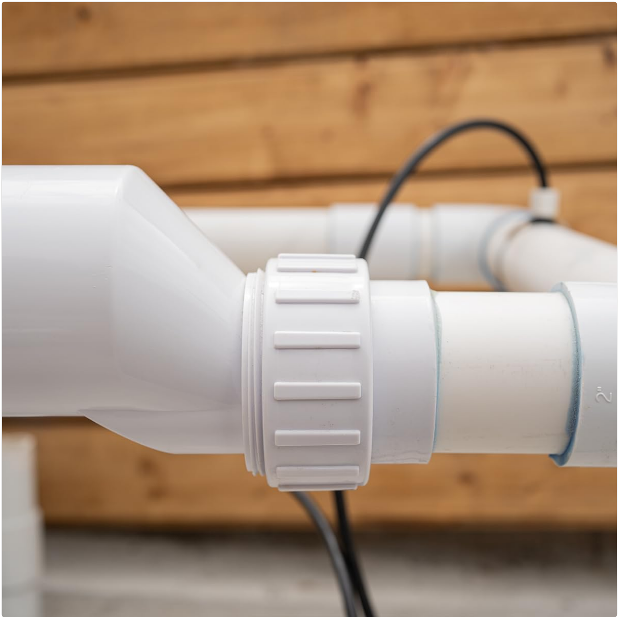
Image: A detailed view of a threaded plumbing connection, part of the salt chlorinator installation, showing secure fitting.
