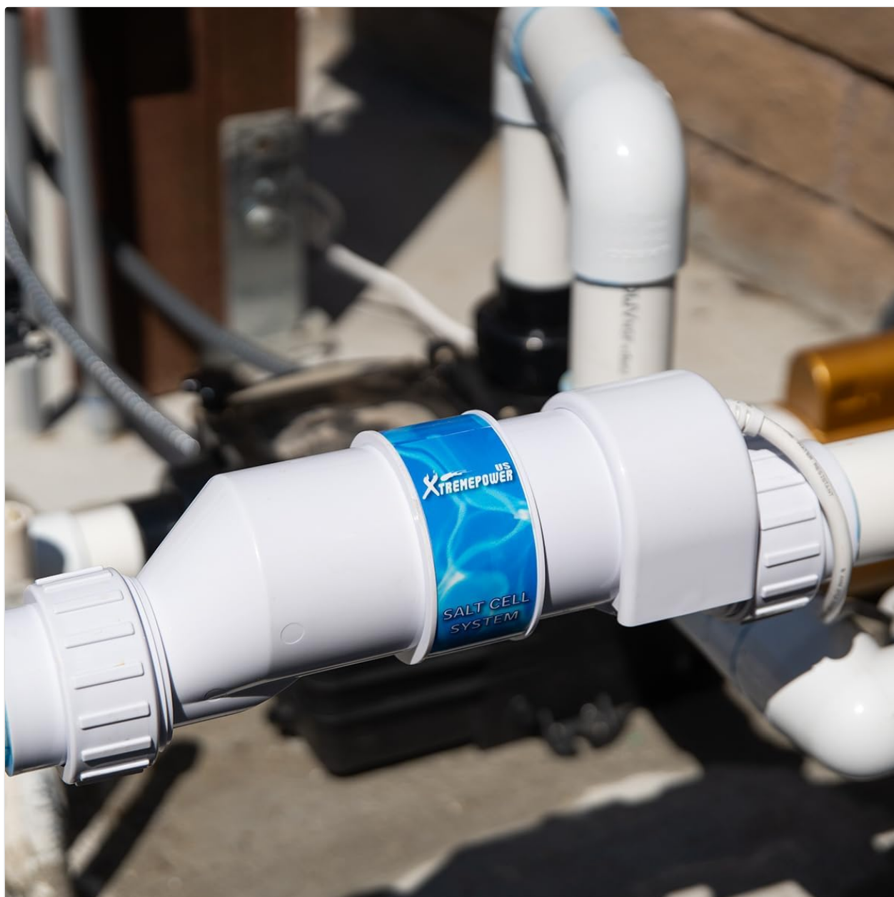
Image: A close-up view of the XtremepowerUS salt cell system integrated into the white PVC plumbing of a pool filtration system.
