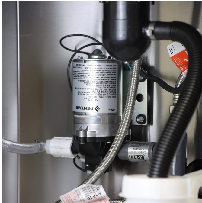
Figure 3: Water pump and plumbing connections.
