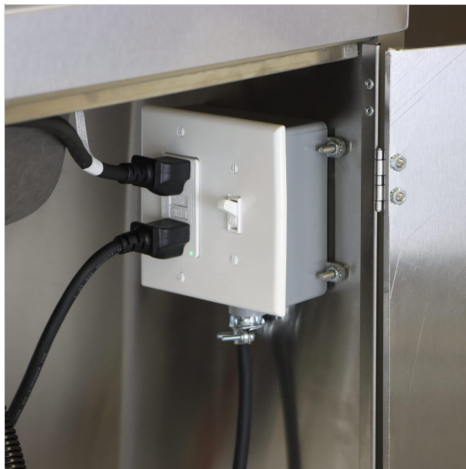
Figure 4: GFCI electrical outlet.
