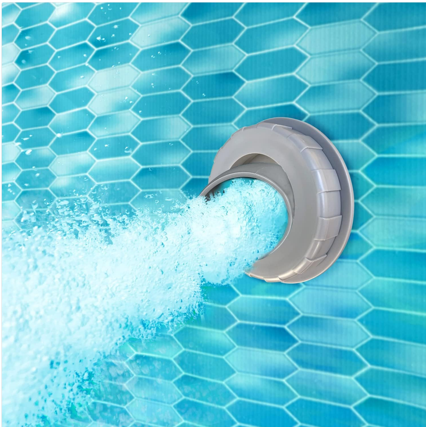
Image 5.2: Filtered water being returned to the pool, illustrating the pump's circulation function.
