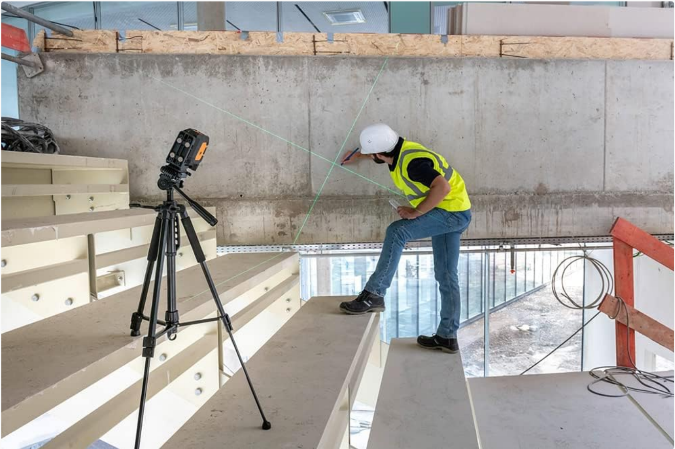
Figure 5: An individual utilizing the GEO1X-GREEN laser mounted on a tripod to project angled lines along a staircase. This demonstrates the device's capability for manual mode operation, allowing for non-level alignment tasks.
