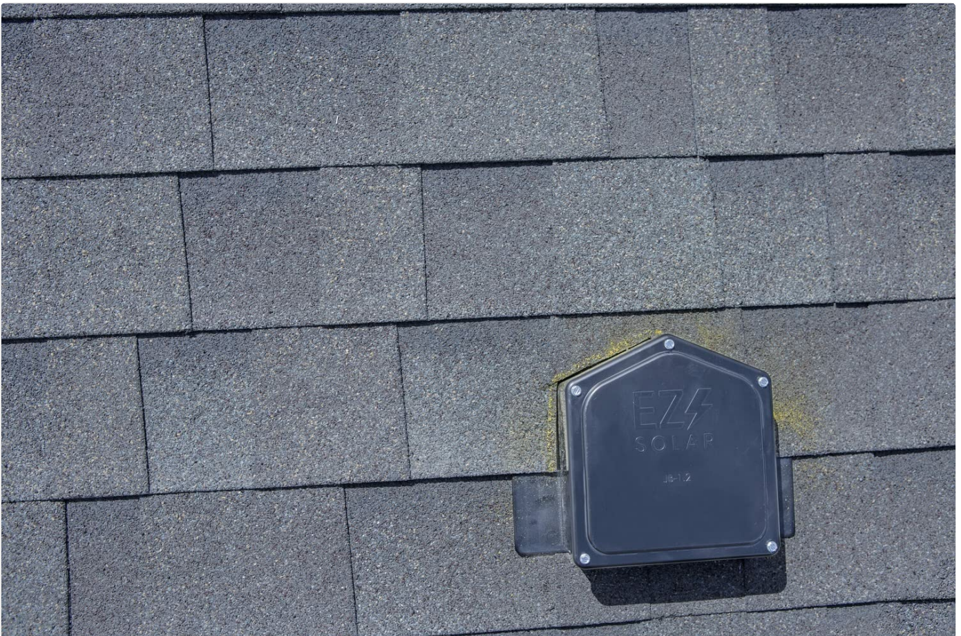
Figure 5.8: The JB-1.2 junction box fully installed and sealed on a shingle roof, blending with the surroundings.
