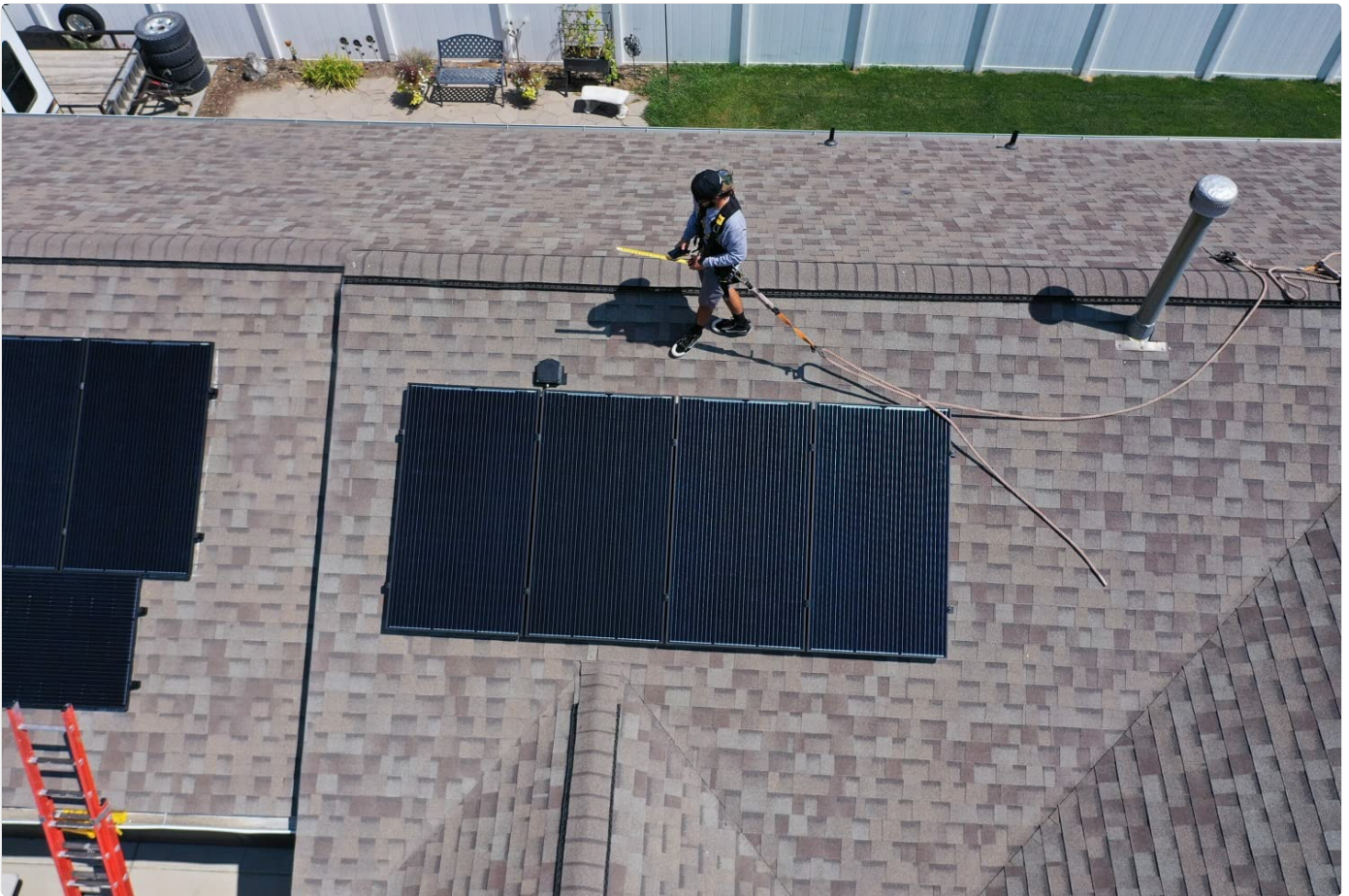
Figure 5.1: Overview of a rooftop solar installation, showing the context for junction box placement.
