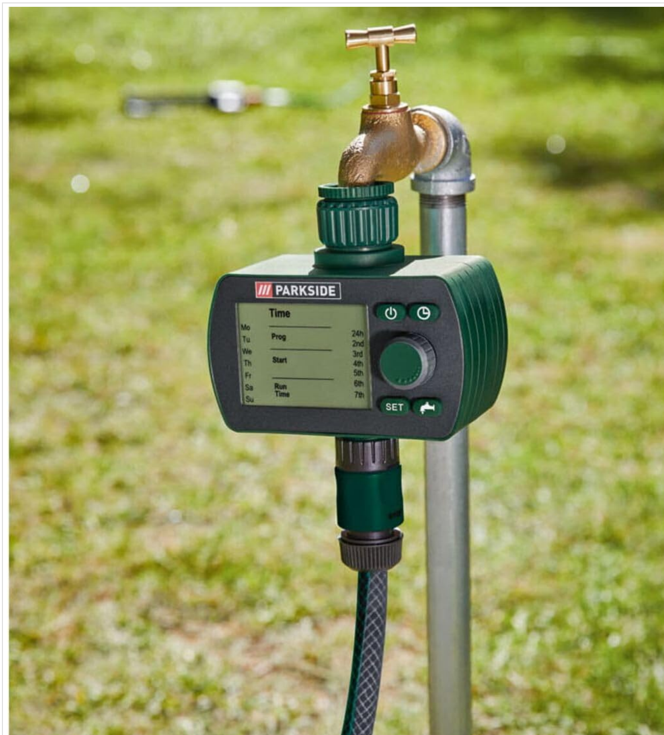
Figure 4: The irrigation programmer properly installed on an outdoor tap, ready for hose connection.
