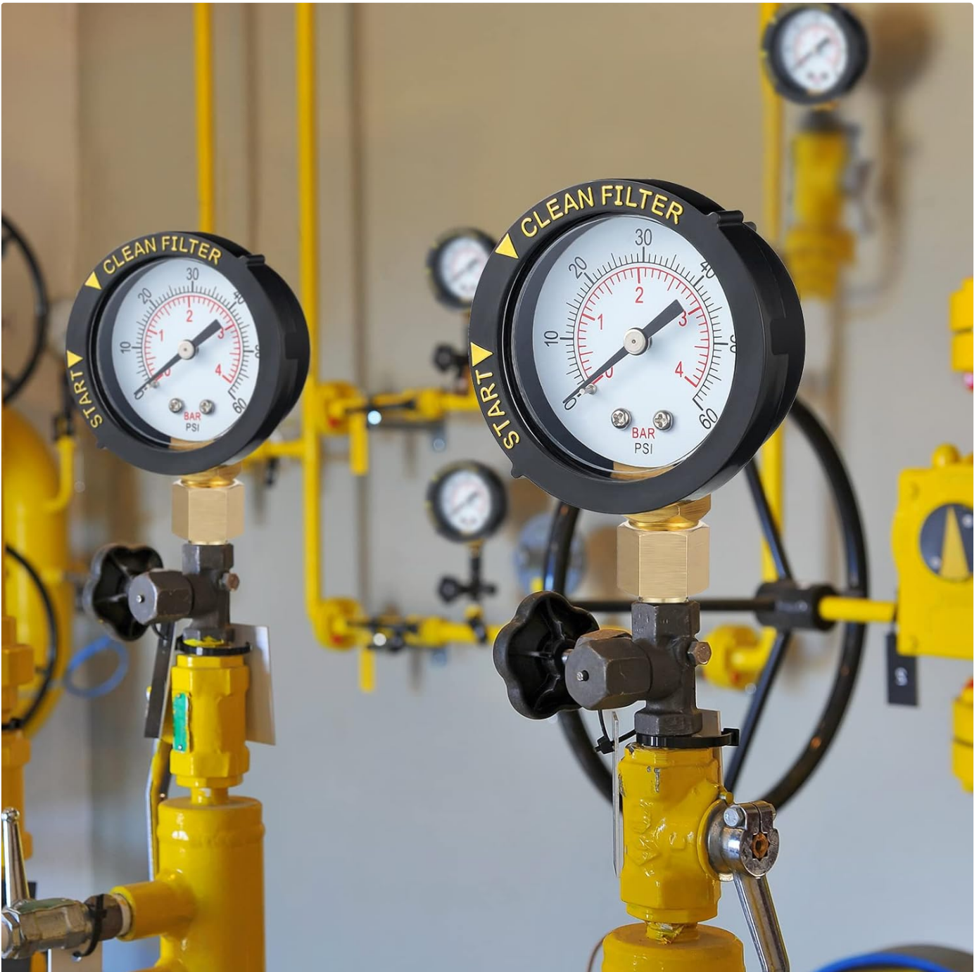
Figure 6: Example installation of the pressure gauges on a filtration system.
