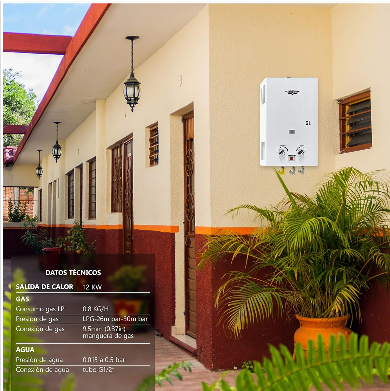
Figure 4: Example of an outdoor installation (sheltered) with technical data.
