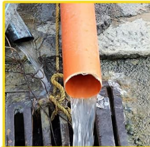
Waste Water Drainage
