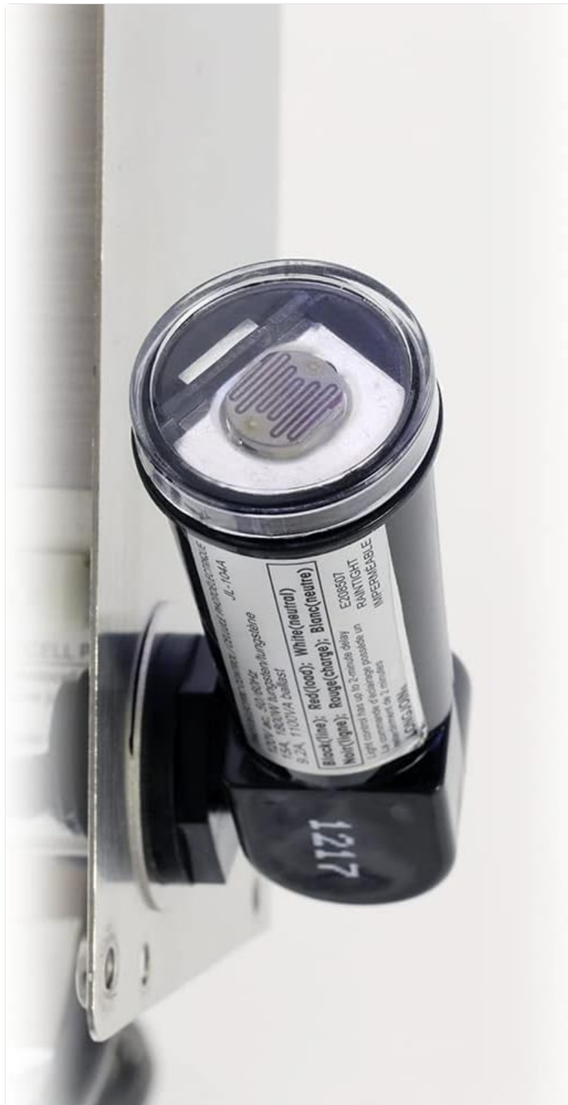
Figure 4: Photocell installed on the transformer.
