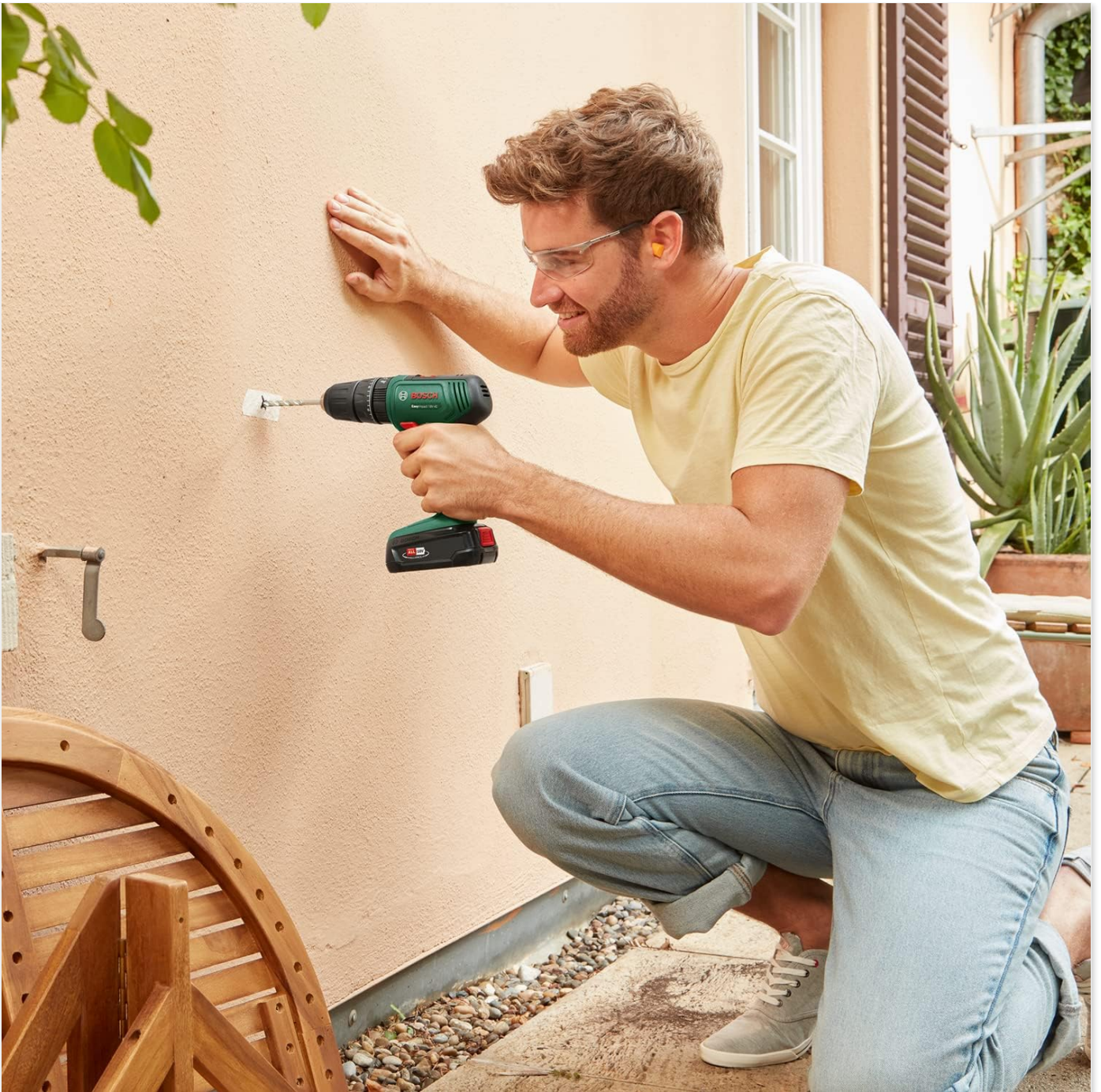
Demonstration of the drill being used for masonry work on an exterior wall.
