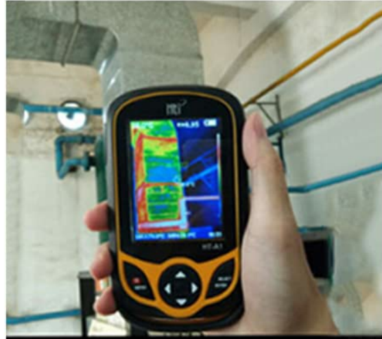
Check exhaust system
