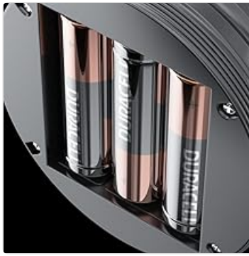
Image: Proper battery installation in the lantern.
