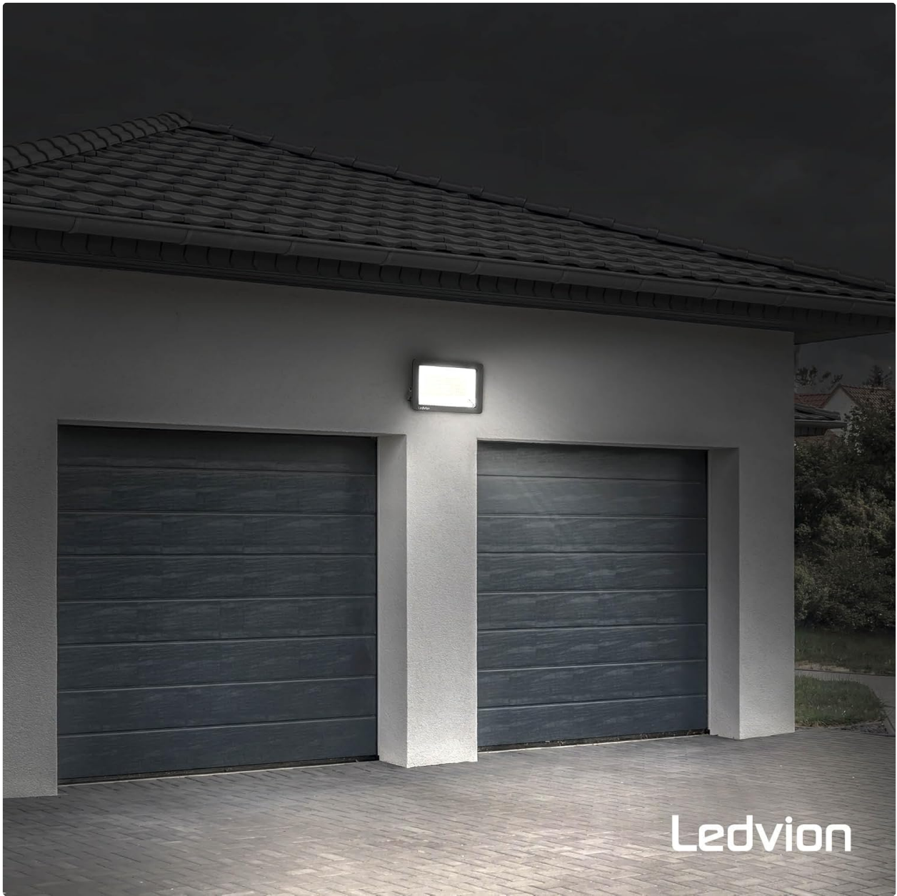
Figure 3.3: Example of the Ledvion floodlight installed for outdoor illumination.
