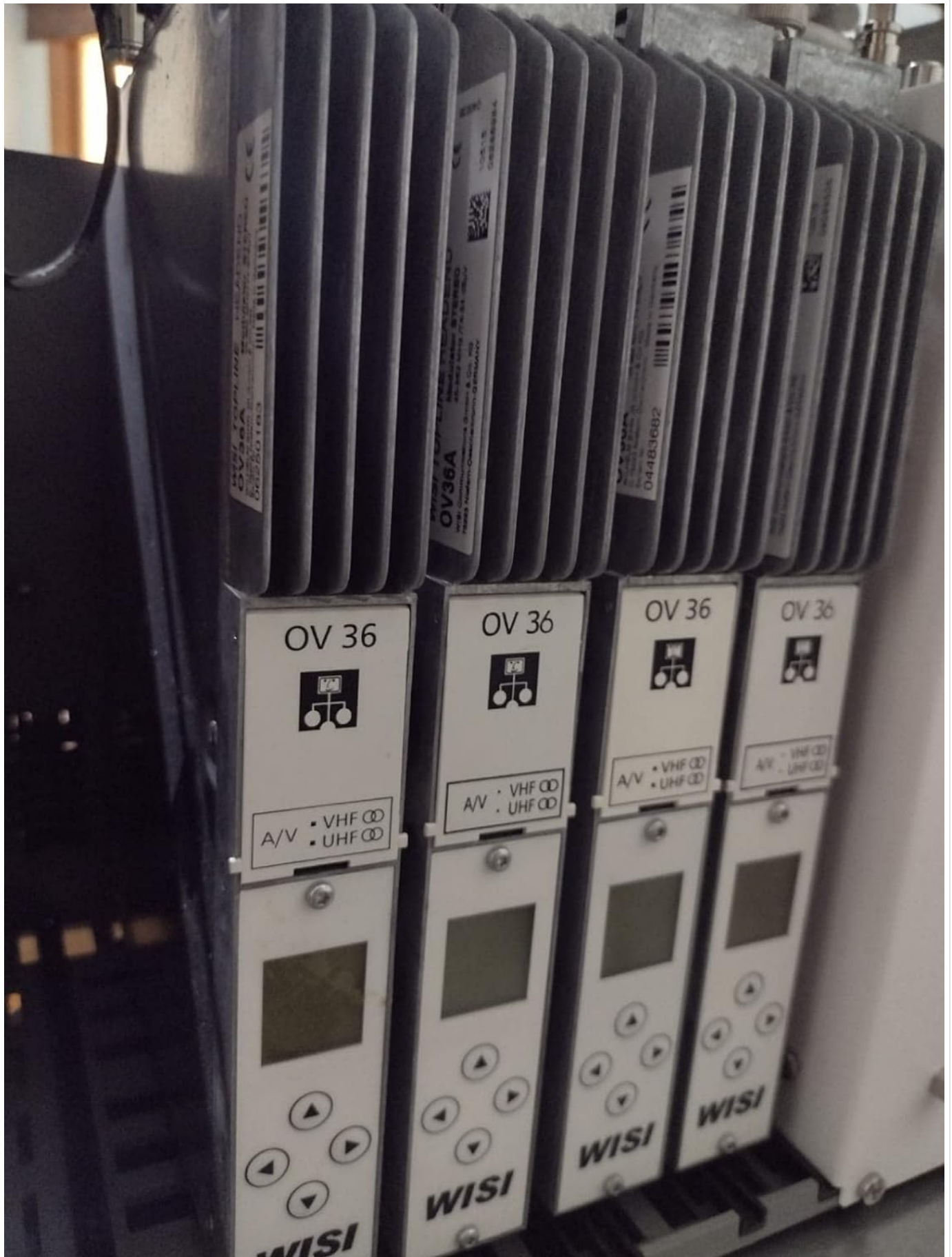
Figure 4.4: Multiple WISI OV36 modules installed in a rack. This image demonstrates the modularity of the system, showing several processing units side-by-side within a larger setup. Serial numbers like 044836 and 06250183 are visible on the modules.
