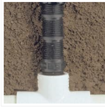
Image: An Orbit cut-off riser extension installed in the ground, connecting to an irrigation line.
