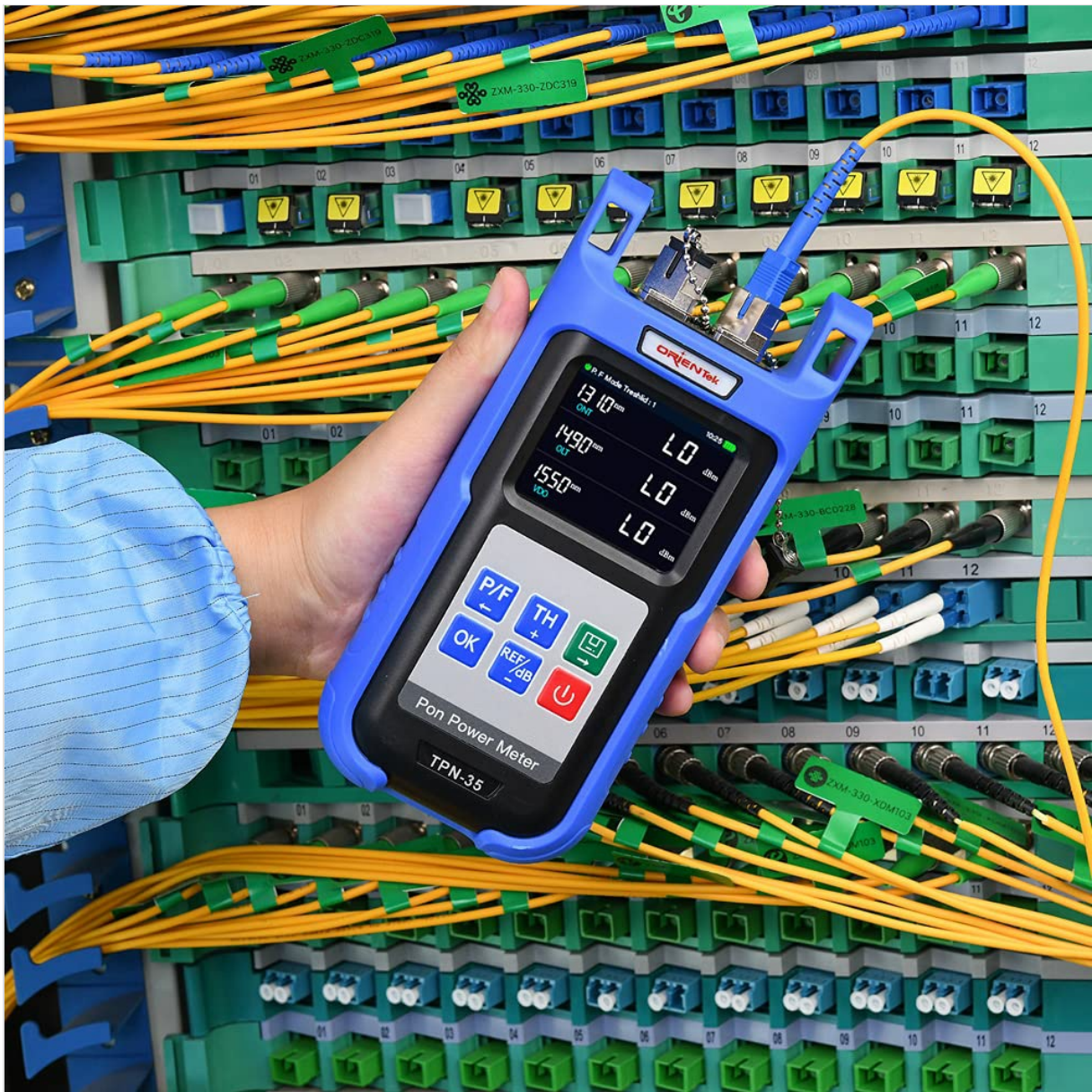
Figure 6: The TPN-35 being used by a technician to test fiber optic connections within a complex network cabinet, demonstrating its application in real-world scenarios.
