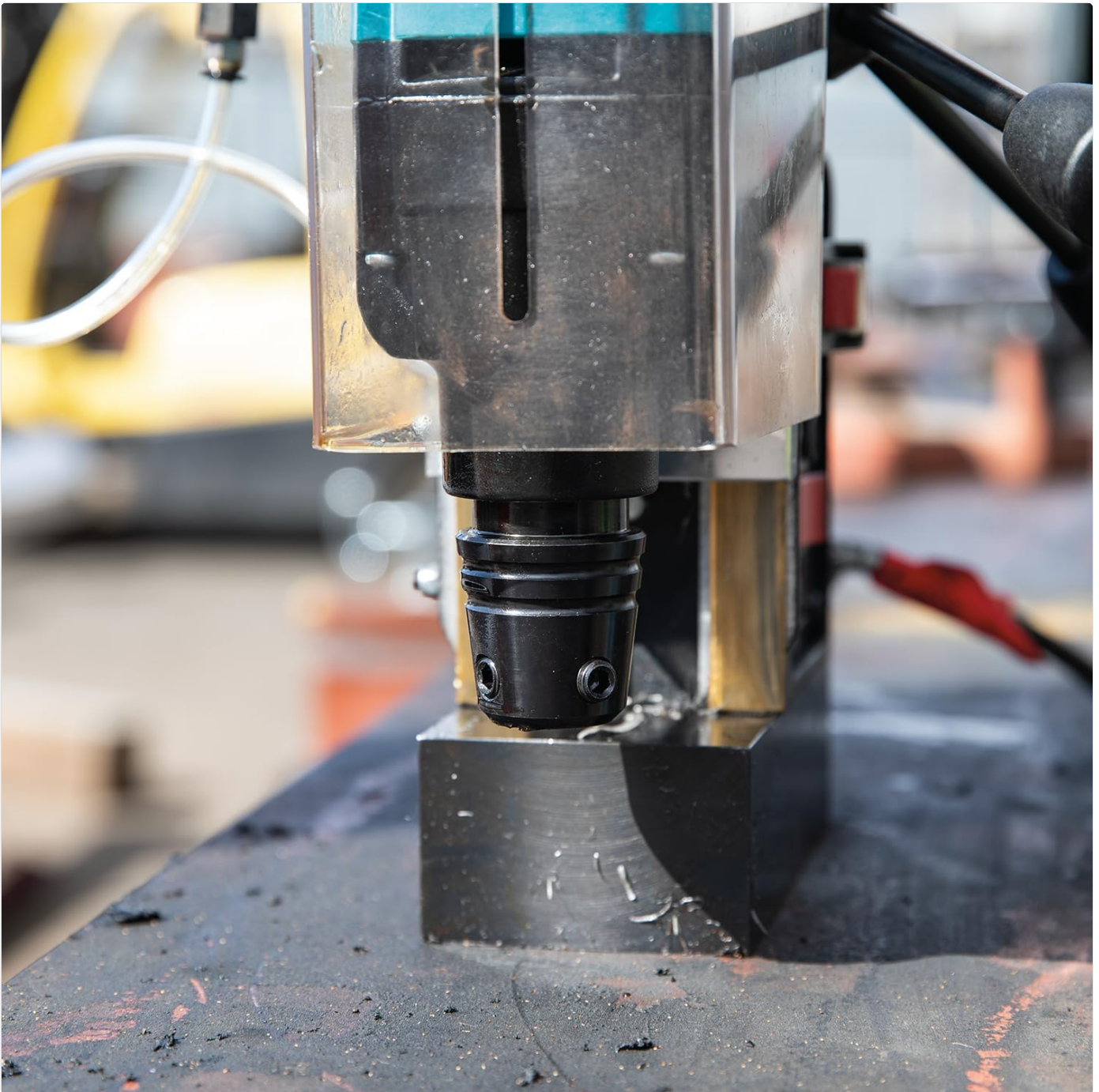
Figure 5.1: The magnetic drill firmly attached to a metal beam, demonstrating proper securing.
