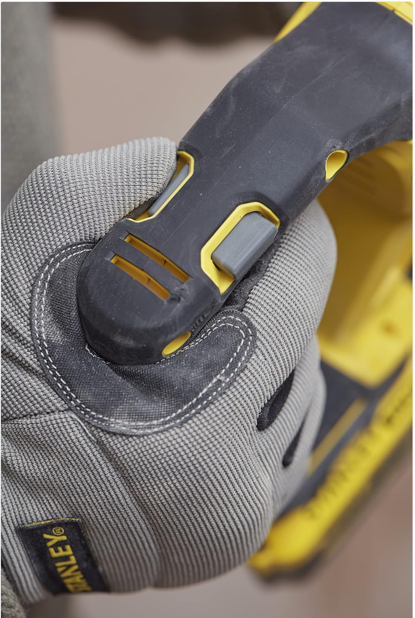
Figure 4.3: A user performing chiseling work with the STANLEY FATMAX rotary hammer, wearing appropriate safety gloves.
