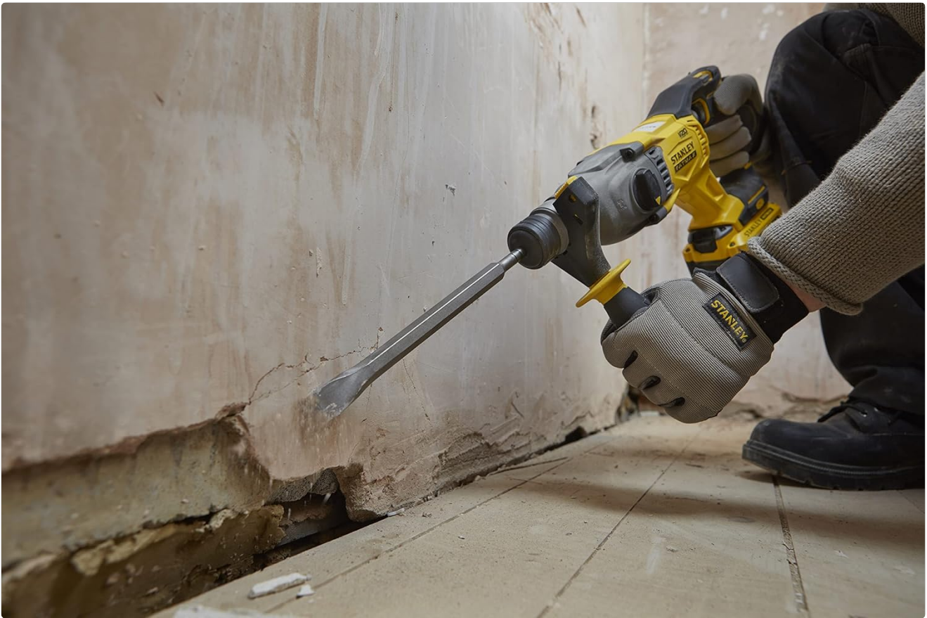
Figure 4.4: Another view of the rotary hammer being used for chiseling, highlighting the tool's impact energy for material removal.
