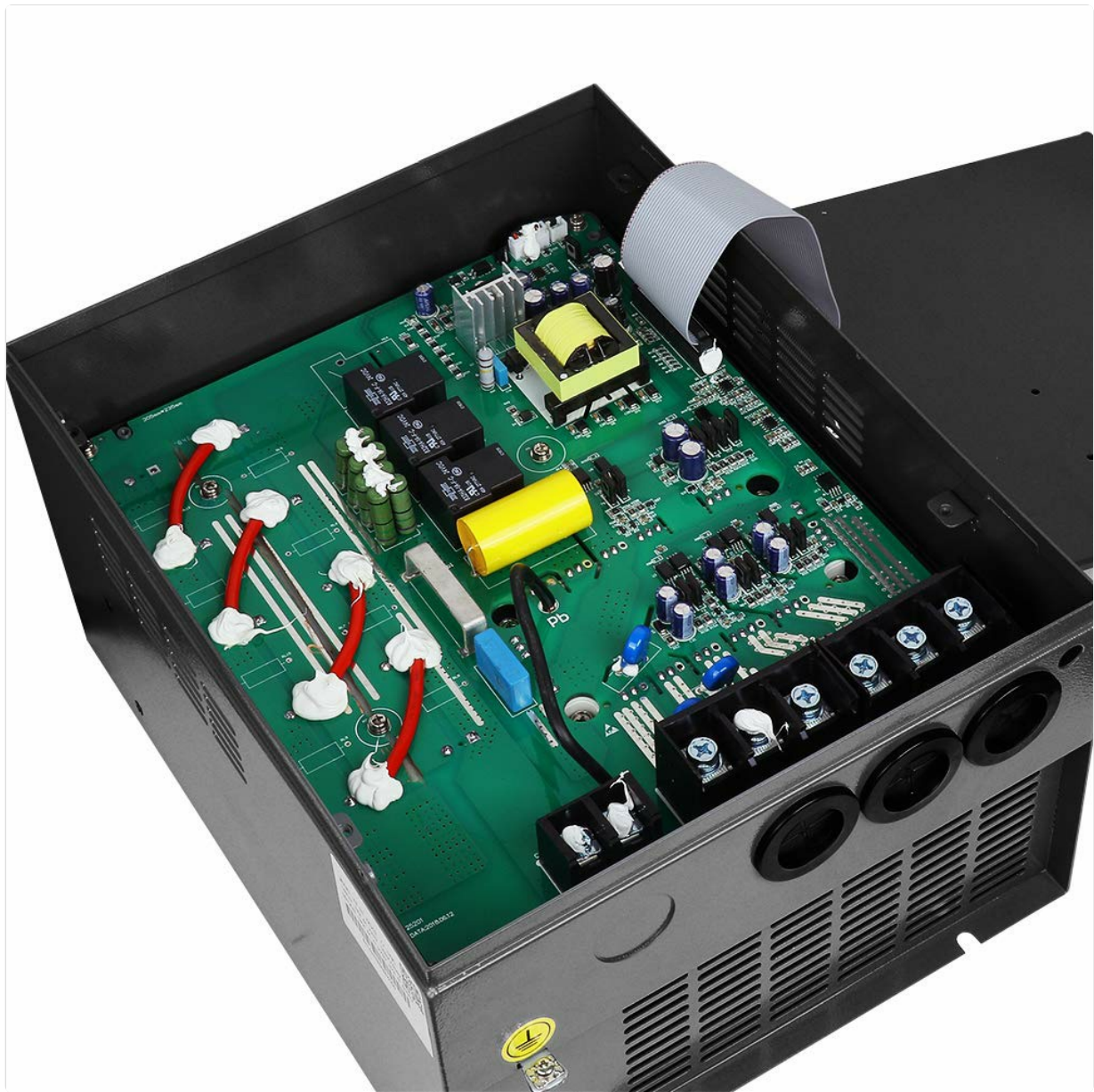
Figure 5.2: Internal view of the VFD, showing the main circuit board, power components, and terminal blocks for input, output, and control wiring. Note the clear separation of power and control sections.
