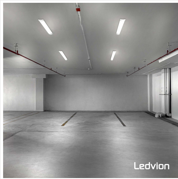
Image: Example installation in a garage.
