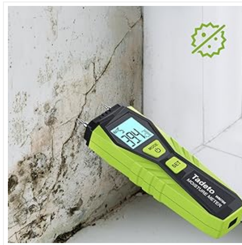
Figure 7: Detecting moisture in a wall, indicating potential water leaks or dampness.
