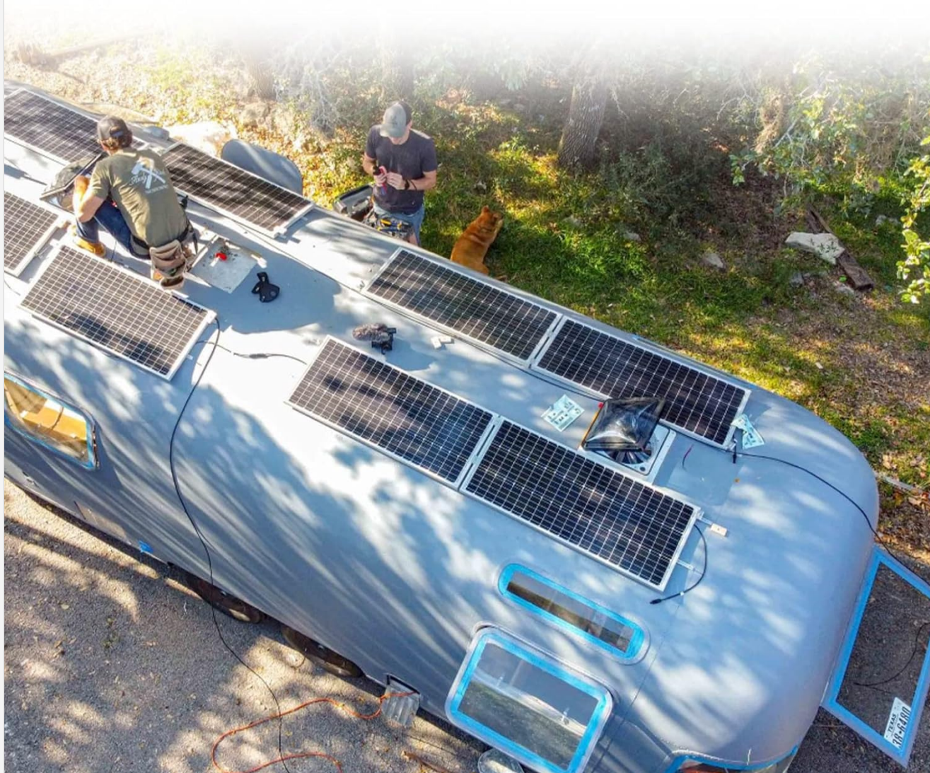
Image 4.1: An RV equipped with multiple flexible solar panels, demonstrating the system's capacity to generate power.
