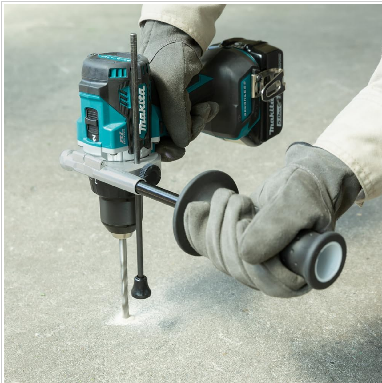
Figure 2: Proper use of the auxiliary side handle for enhanced control during drilling.
