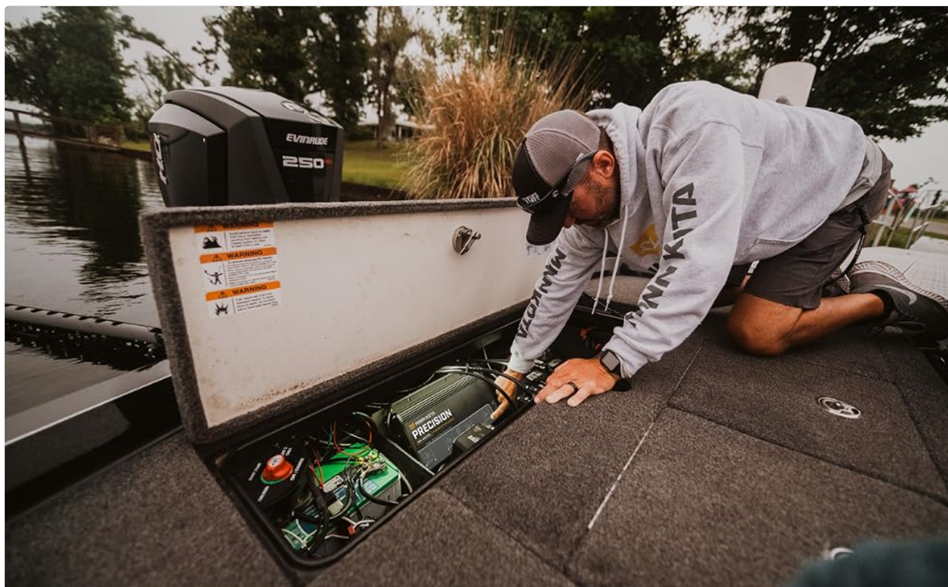
Image: Minn Kota Precision Charger MK 230 PCL installed in a boat's battery compartment. This image shows the charger mounted within a boat's storage area, connected to batteries.
