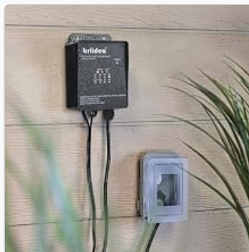
Image 6.2: The transformer mounted on an exterior wall, demonstrating a typical installation scenario.
