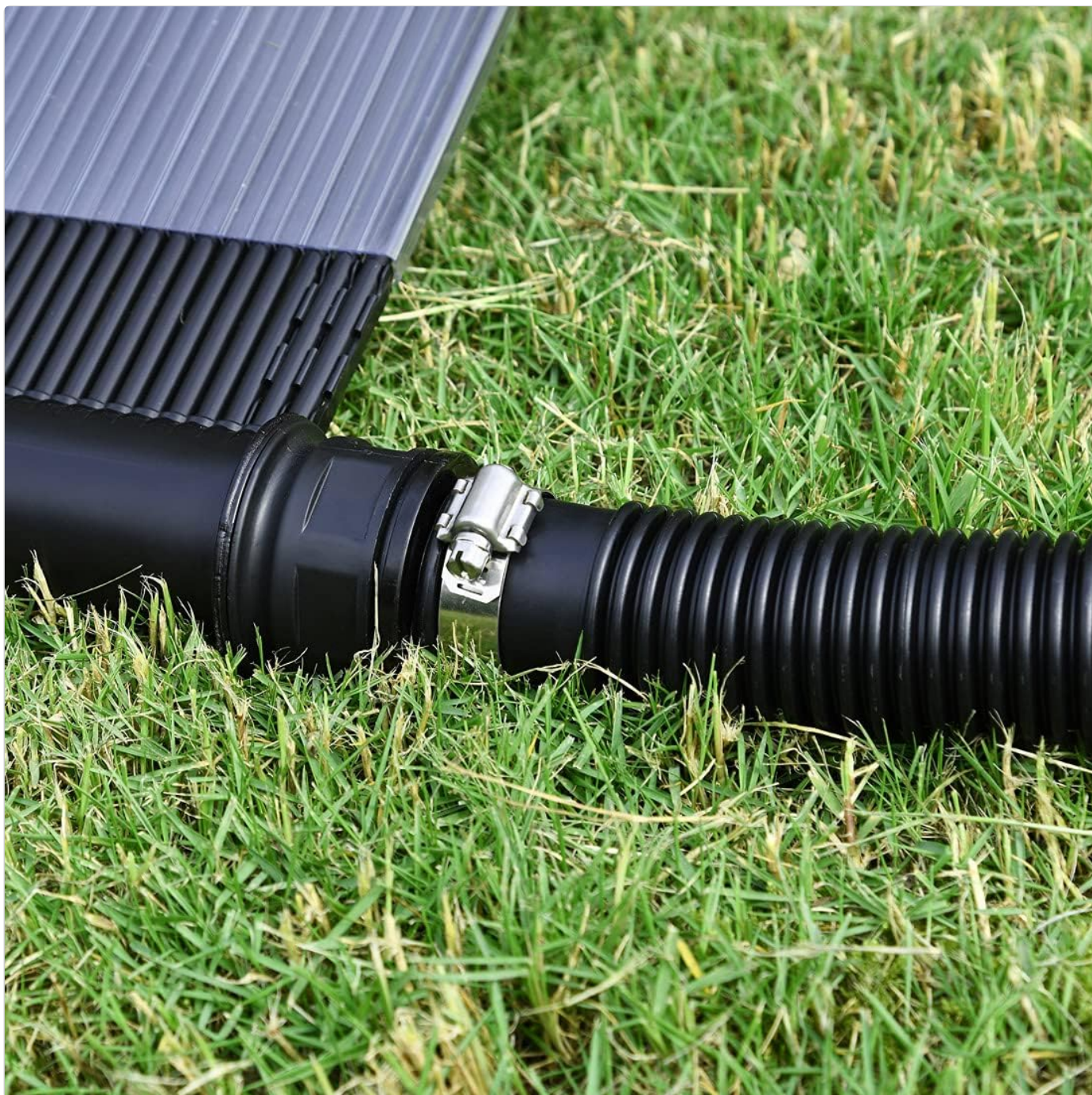
Image: Detailed view of a hose securely connected to the solar panel using a stainless steel clamp, ensuring a leak-free connection.
