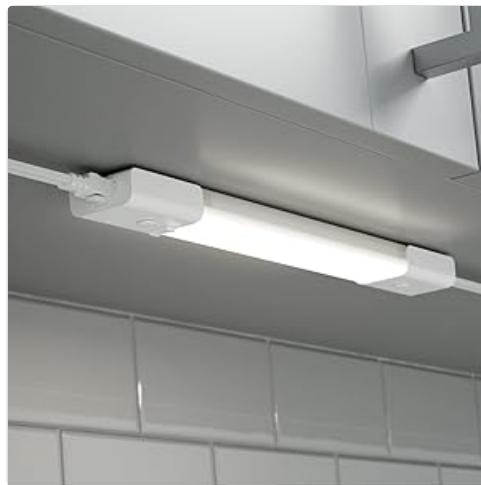
Image: A close-up of the GE LED HD+ Undercabinet Light Fixture installed and emitting light, showcasing its slim profile and effective illumination of the kitchen backsplash.
