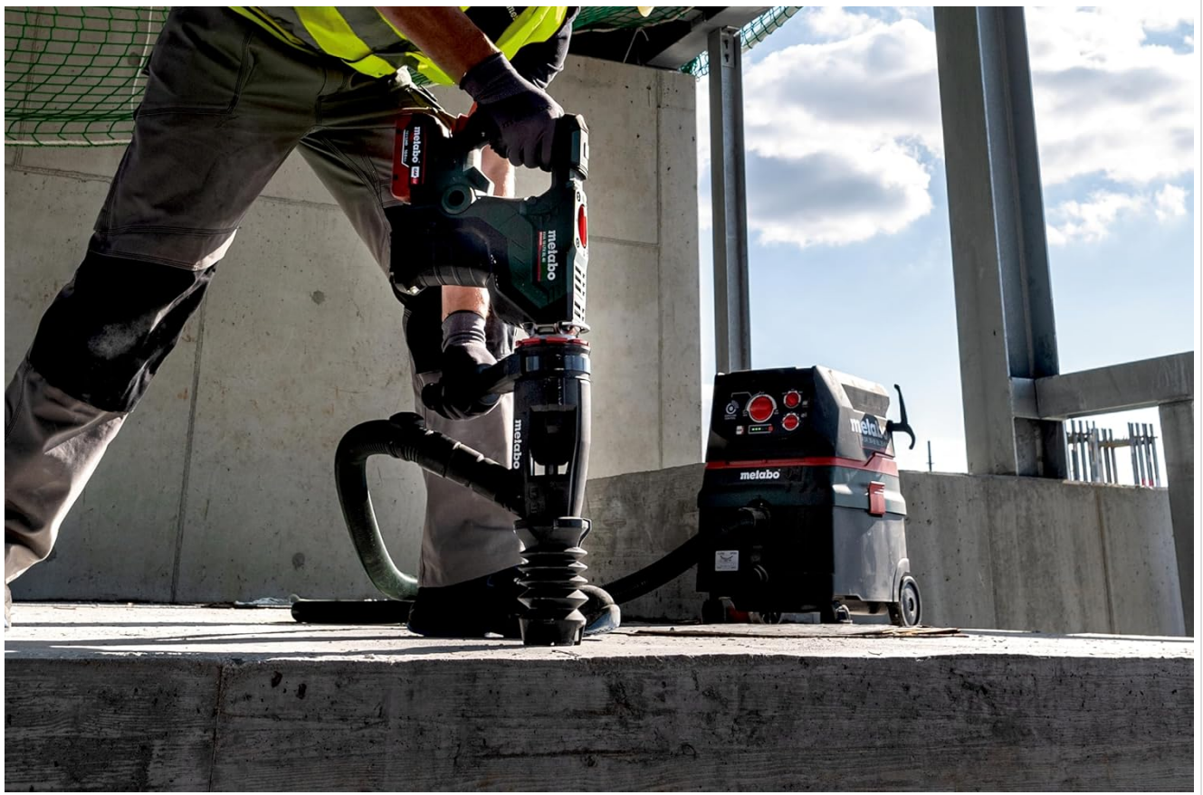
Figure 4.1: A worker operating the Metabo KHA 18 LTX BL 40 for vertical drilling into a concrete surface, utilizing an external dust extraction system for a cleaner work environment.
