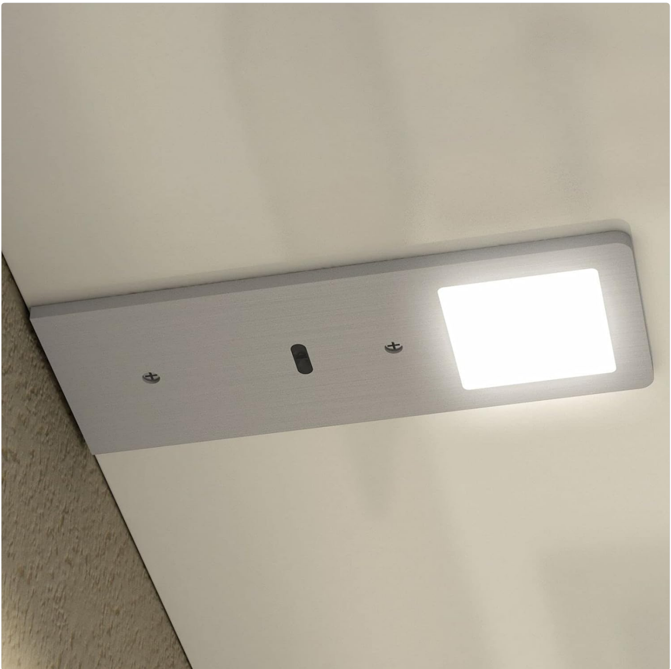
Image 4.3: Close-up view of the installed LED light, showing the sensor.
