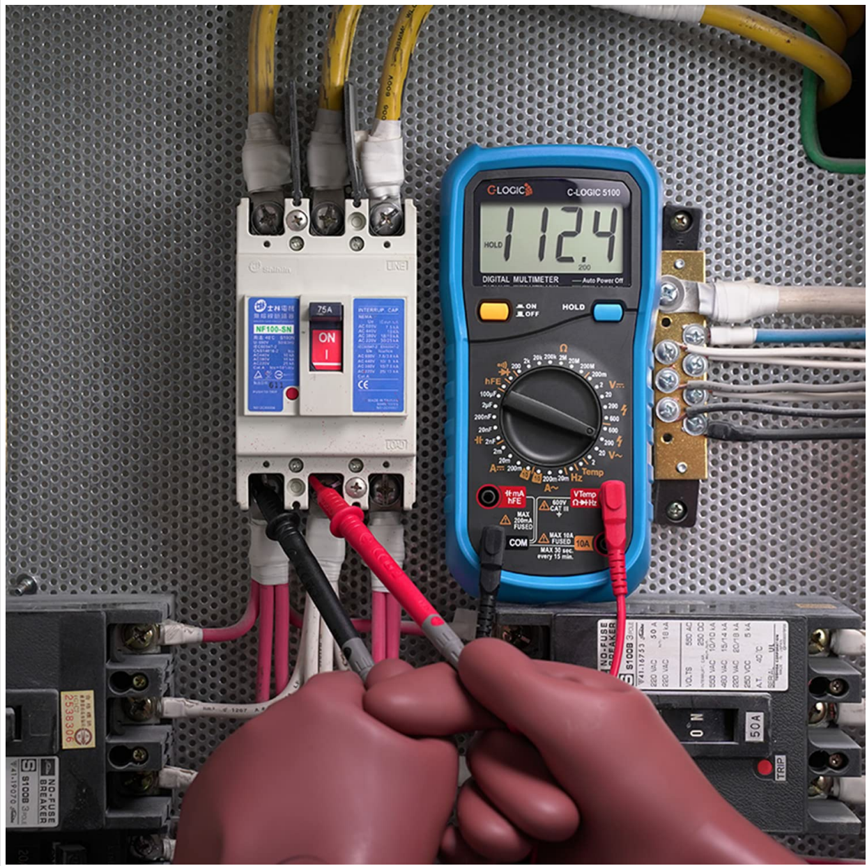
Figure 2: The C-LOGIC 5100 Digital Multimeter actively measuring voltage in an electrical panel.
