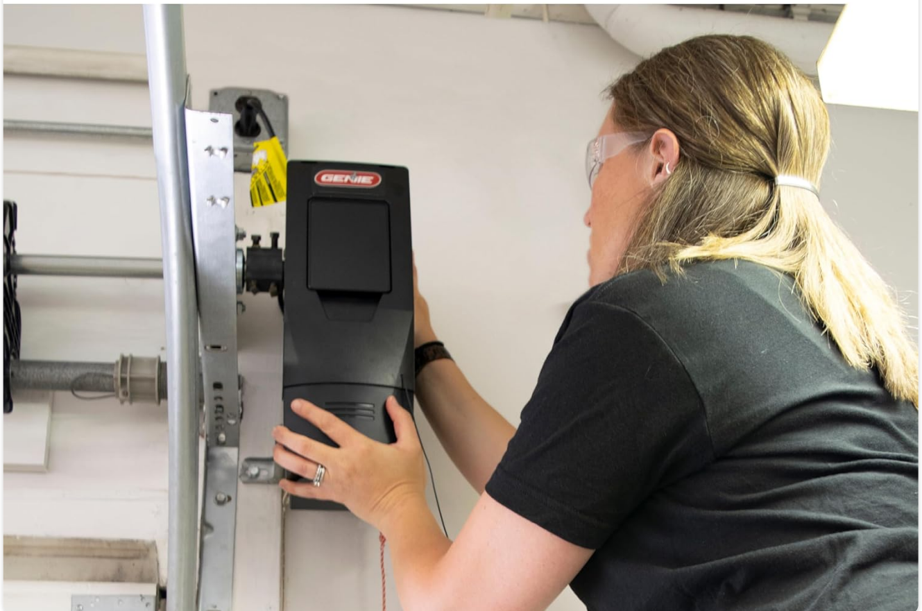
Figure 10: Illustration showing the Genie garage door opener functioning during a power outage, thanks to its integrated battery backup system.
