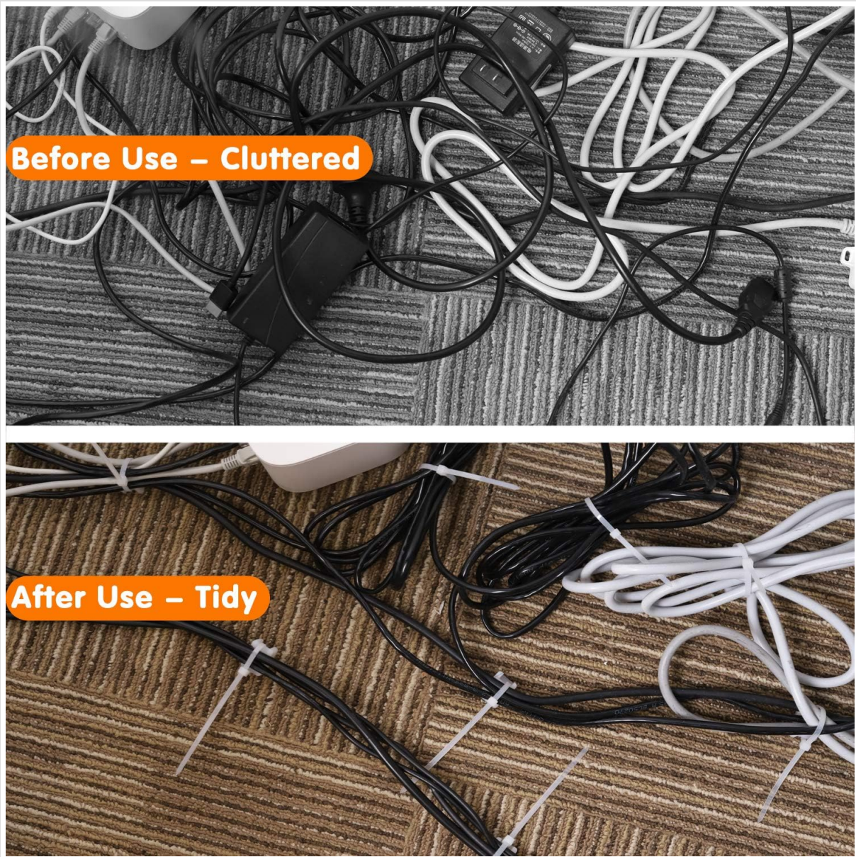
Image: A visual comparison showing a cluttered area of cables before organization and the same area after being tidied with cable ties.
