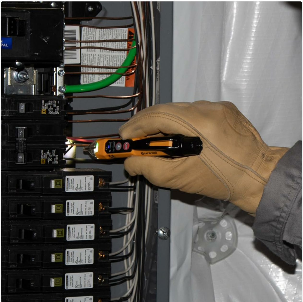
Figure 8: Using the NCVT3P to detect non-contact voltage.
