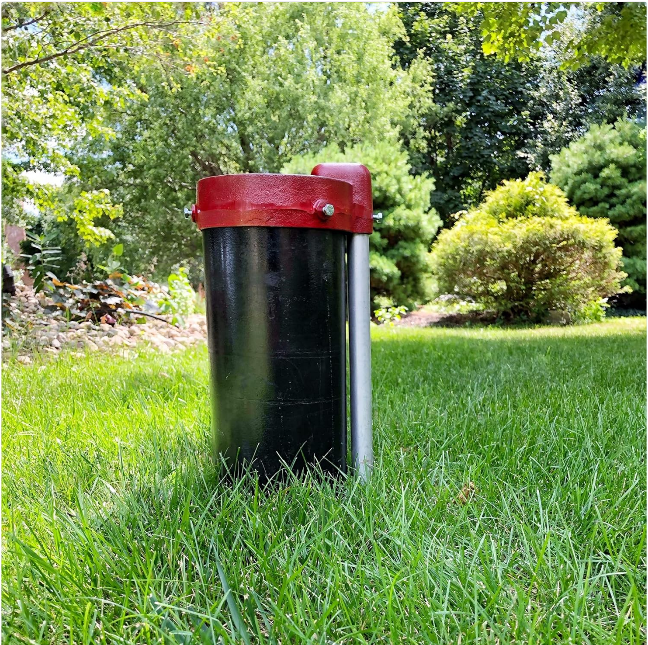
Figure 5: A closer view of the installed well cap, illustrating how it fits over the well casing and the conduit connection.
