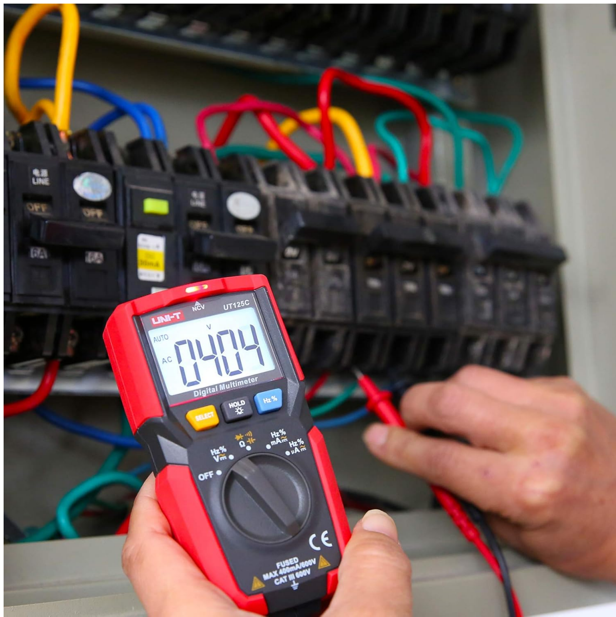
Figure 6: The UT125C Multimeter being used to measure voltage in an electrical panel.
